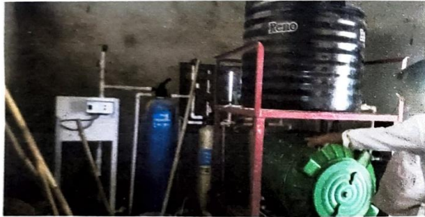
Water purifying RO unit
