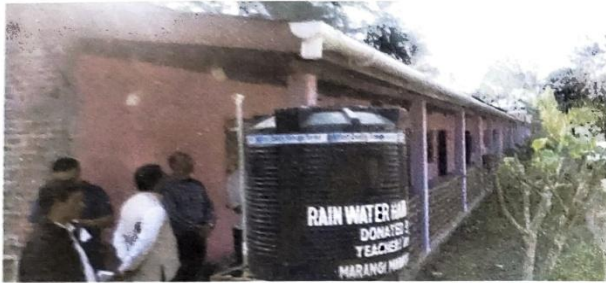
Rain Water harvesting tank
